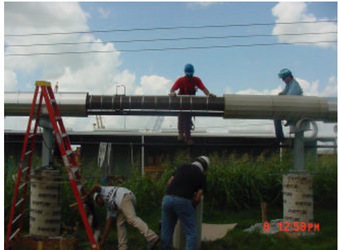
4 KM (13K FT.) OF 12-INCH SULFUR PIPING COURTESY CARGILL INC.
