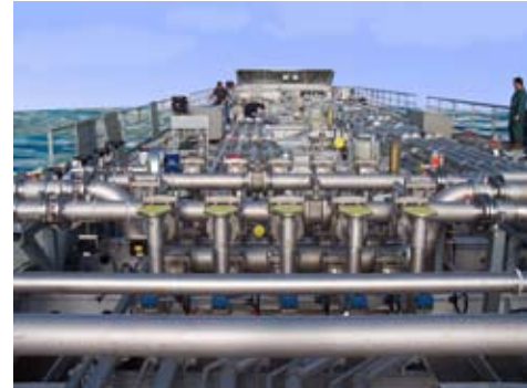
Tanker deck overview
